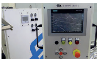
Main operating panel.
